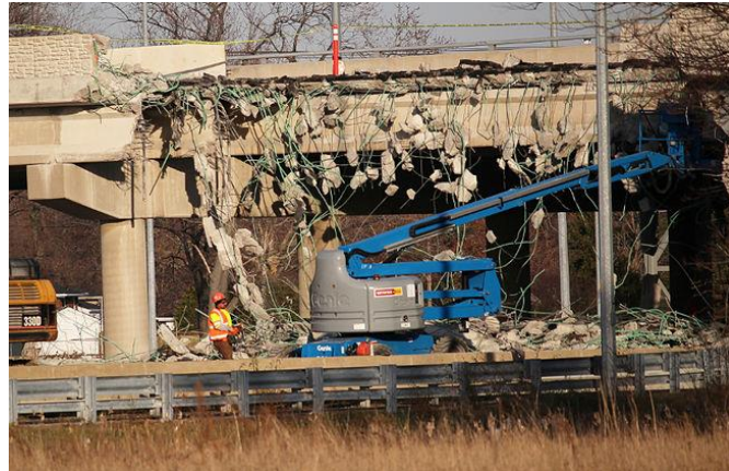
Figure 2-1: Repairs to Hwy 402 Bridge from Oversize Vehicle
