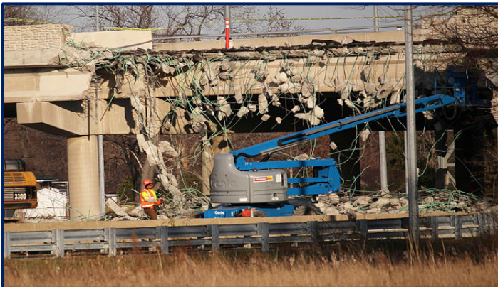
Damage to Provincial Infrastructure:
