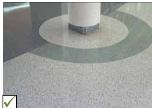
Where a structural column / support may be within an accessible route, a colour contrasted floor surface at base helps identify its location to prevent a potential bumping hazard.
