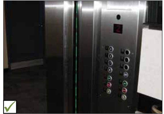
Elevator sensor door and floor registration buttons.
