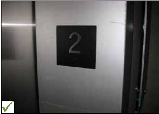
Tactile elevator car identification sign.
